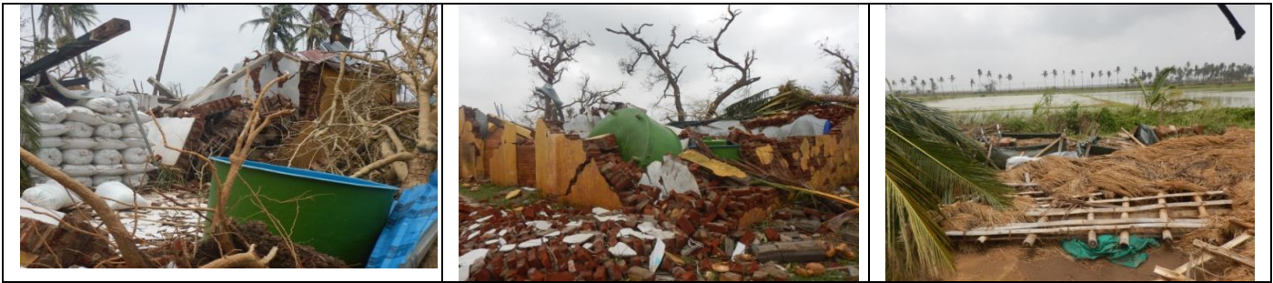
Damage of farm godown and demo units
